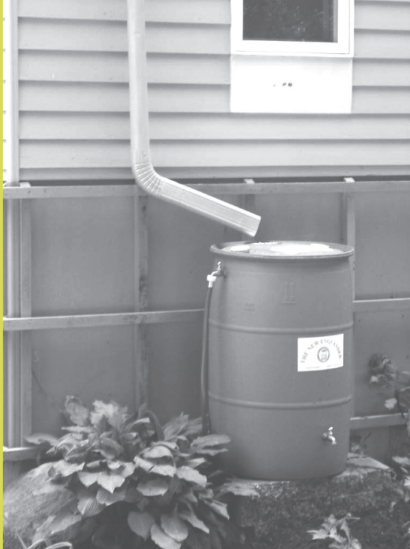
The overflow outlet from this rain barrel drains into an adjacent rain garden. Photo: GeoSyntec Consultants, Inc.
