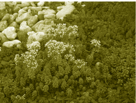
Above, middle: A photo of the green roof at the Bruker Deltronics Headquarters in Billerica, MA. Photo: © 2005, Roofscapes, Inc. Used by permission; all rights reserved.
