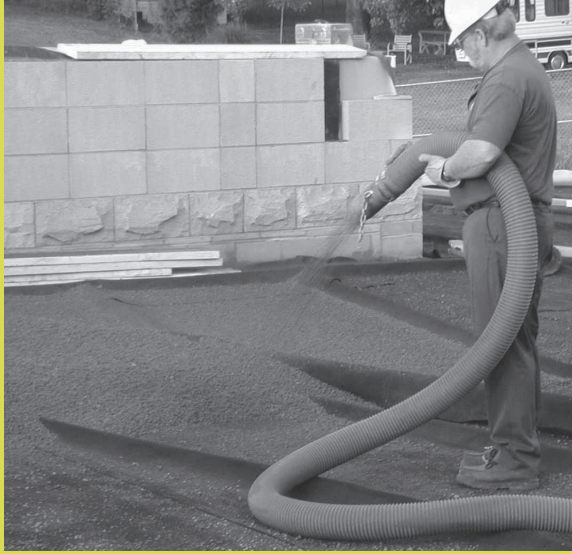
Above: Installation of eight inches of soil medium using pneumatic equipment at the Oaklyn Branch Library in Evansville, IN. Photo: © 2005, Roofscapes, Inc. Used by permission; all rights reserved.
